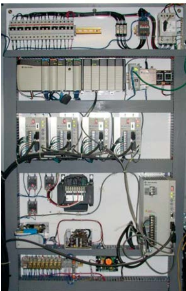
UL approved control panel with multi-axis servo
